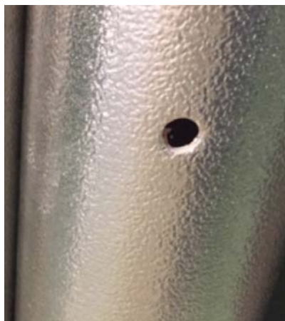
Figure 6: \frac{3}{4} " weep hole drilled into jacketing to promote water drainage from a saturated system
